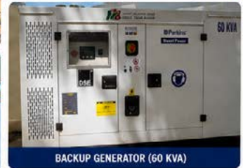
BACKUP GENERATOR (60 KVA)
